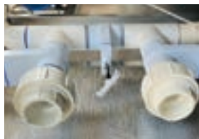
Heat pump ready
